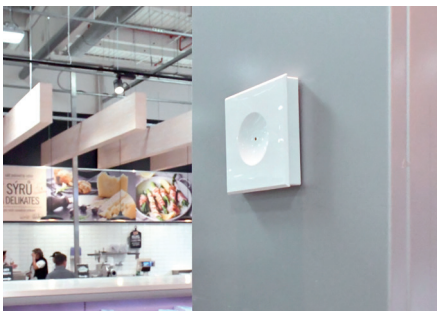
Temperatures and humidity monitoring (lobby) (LS1).
